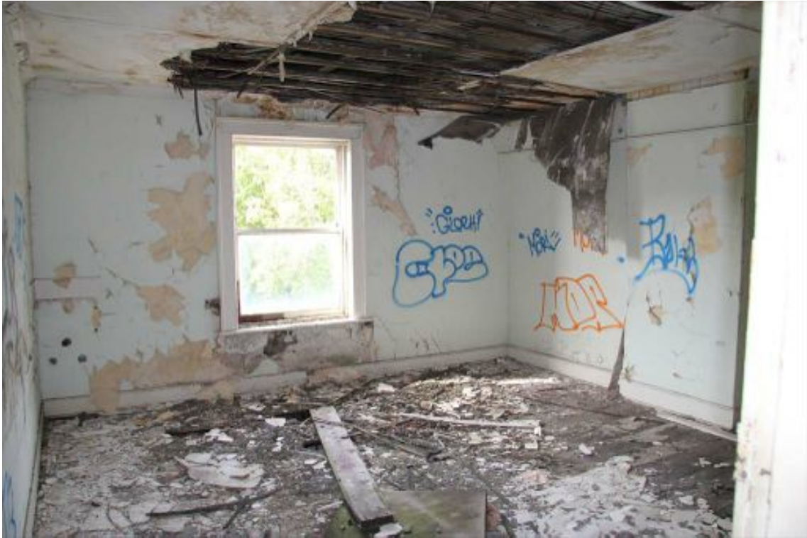
Figure 18 A typical room on the upper level showing collapse of a later fibrous plaster ceiling. Water damage is such that a number of floors have rotted out.
