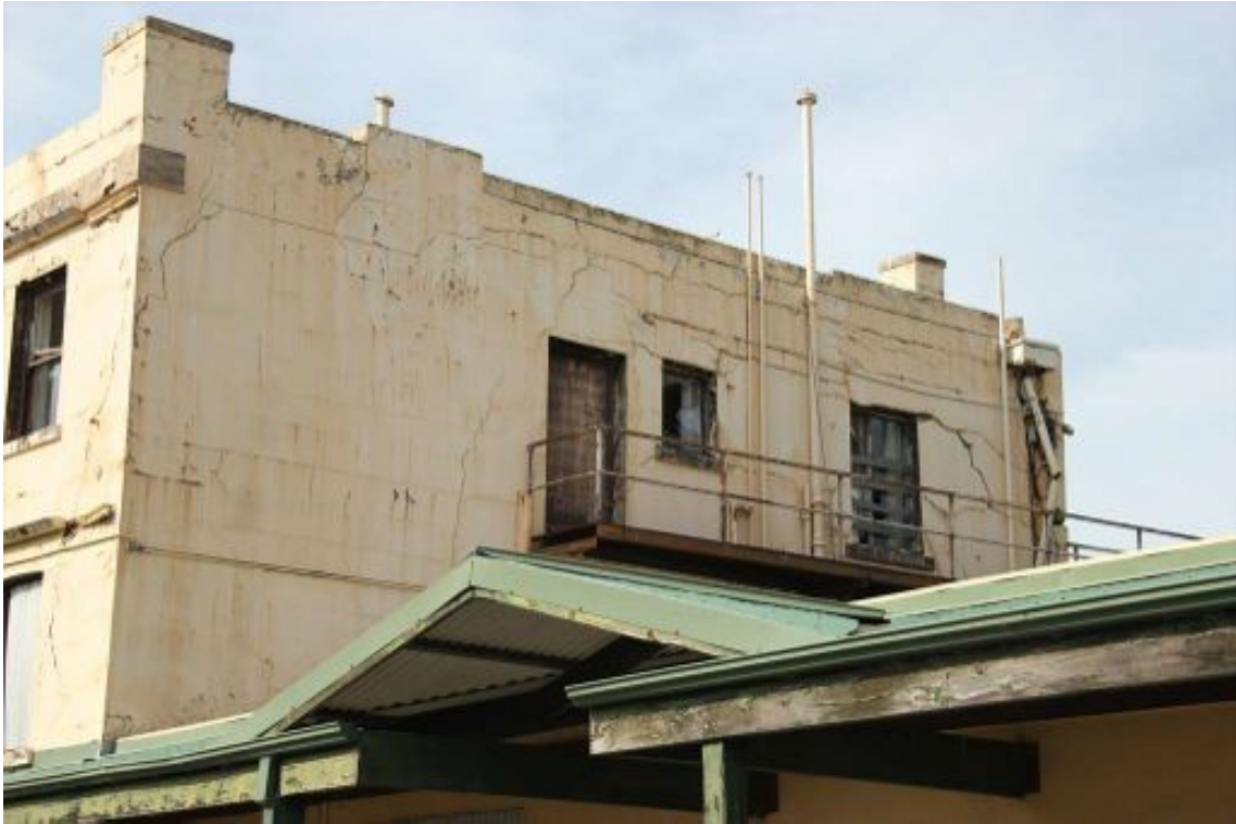
Figure 16 Detail of the south facade showing cracking and deterioration of the rendered finish.
