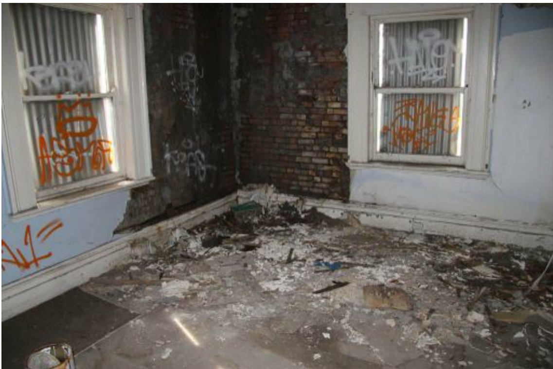
Figure 19 Detail of wall plaster collapse. The detailing of the window sashes confirms that they date from the twentieth century.
