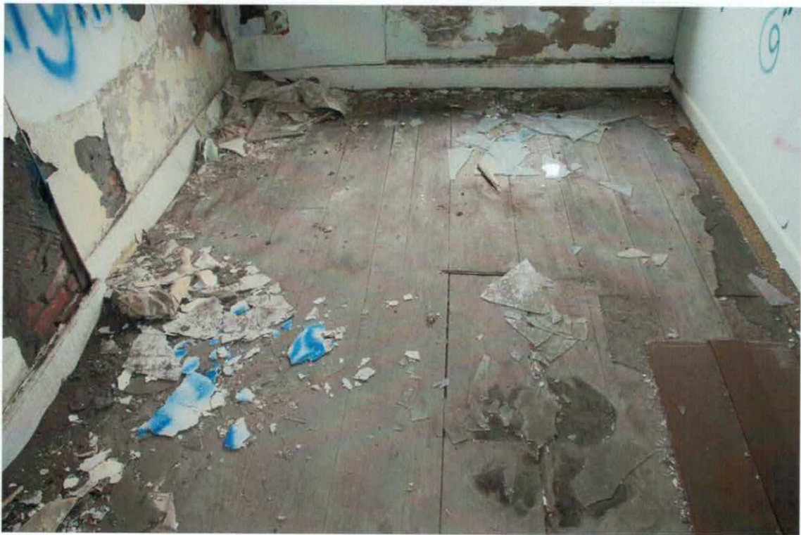
Figure 22 A typical floor showing varying board widths. The boards are tongue and groove jointed.
