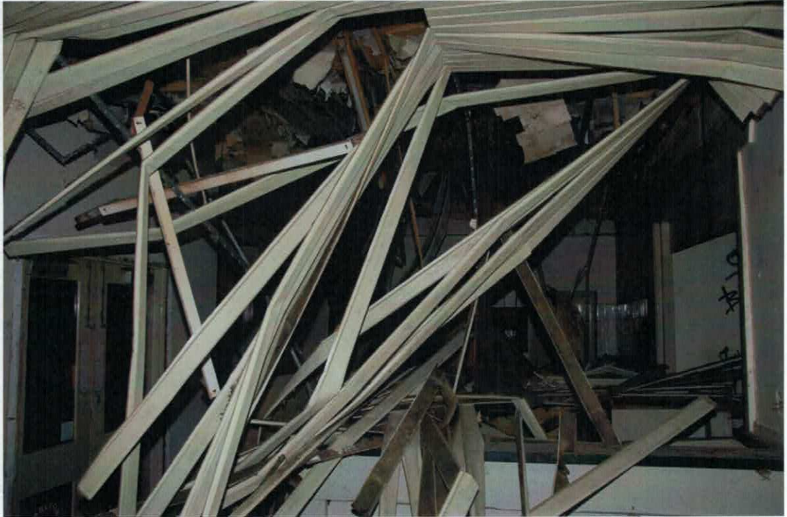
Figure 9 The partially collapsed ceiling and floor structure in the Nelson Place corner bar.
