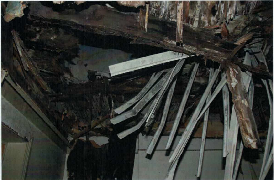
Figure 10 The partially collapsed ceiling and floor structure in the Nelson Place corner bar.
