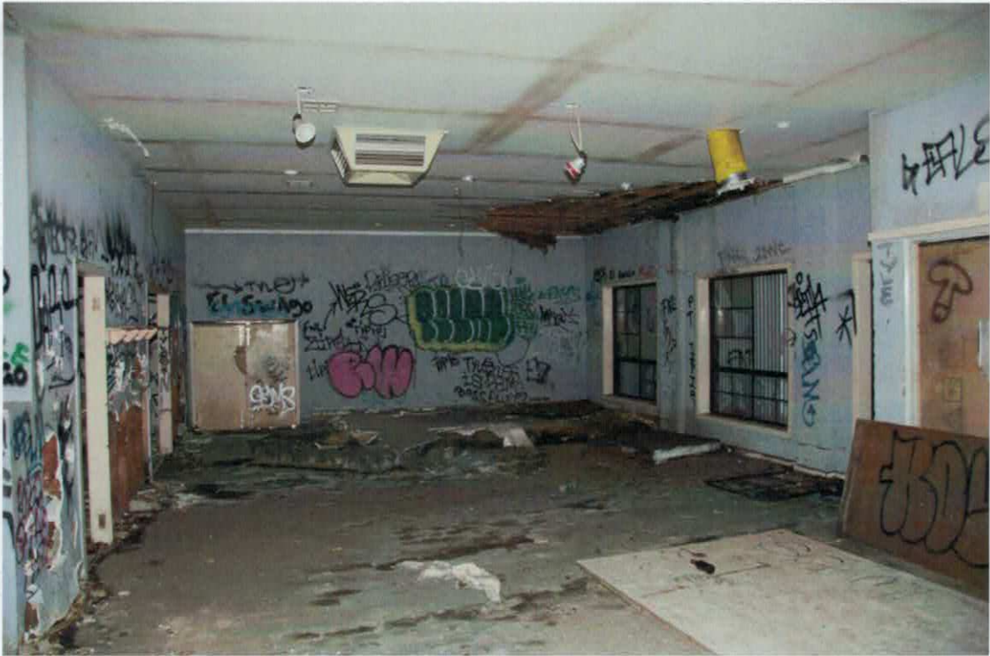
Figure 5 The single storey wing to Ann Street. The physical evidence indicates that the roof framing is of recent origins and that the Ann Street wall is constructed of modern brickwork.
