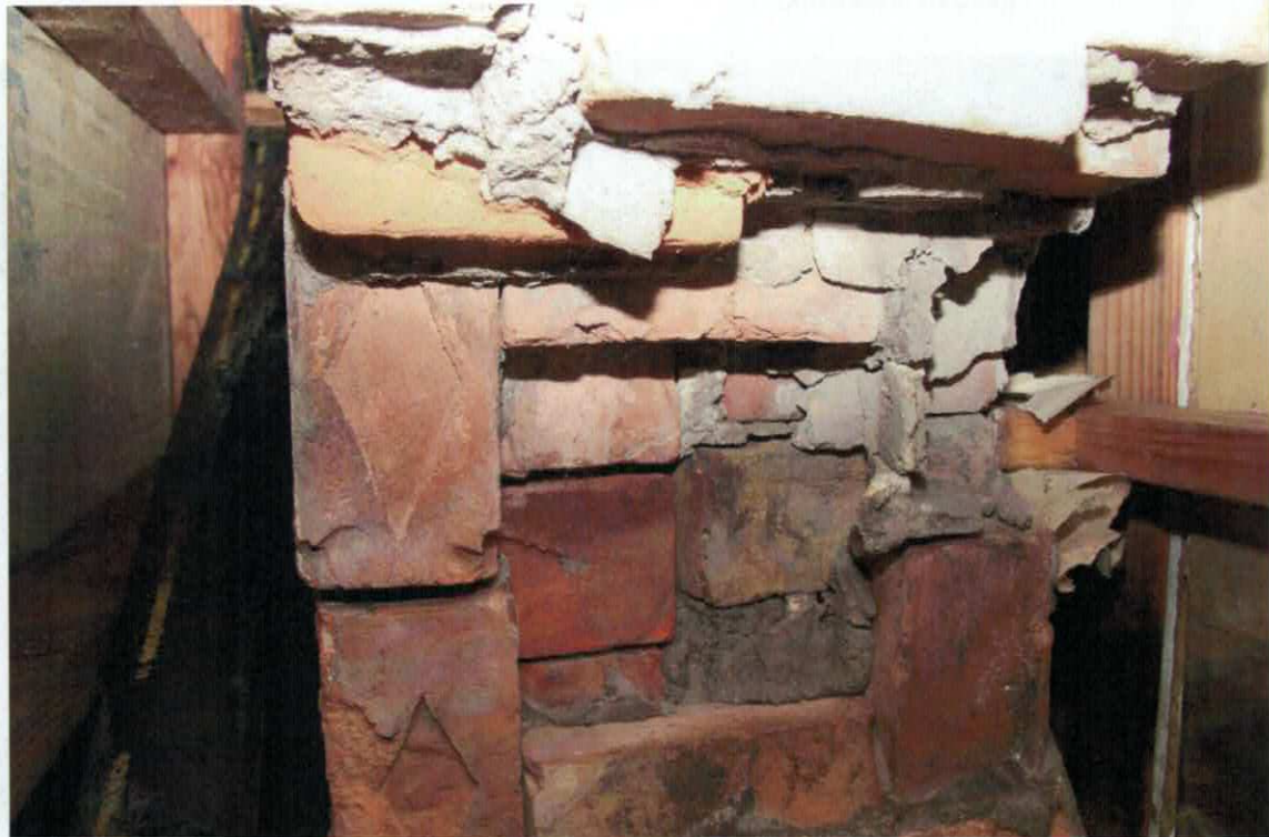
Figure 8 The walls are typically of solid brickwork. A single brick measured at 8" x 3 5/8 th " x 2 1/2 inches. A diamond frog occurs in some bricks. The bricks are as would be expected for the date of construction.
