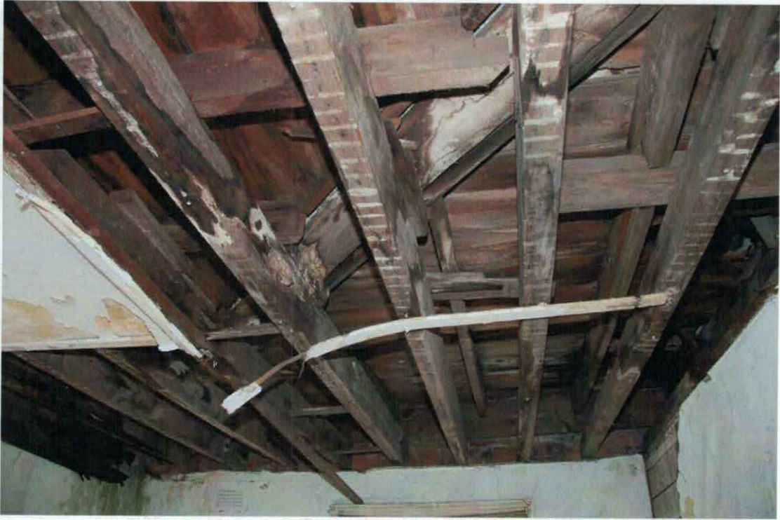
Figure 21 The underside of the roof framing showing the structure supporting the earlier flat roof.
