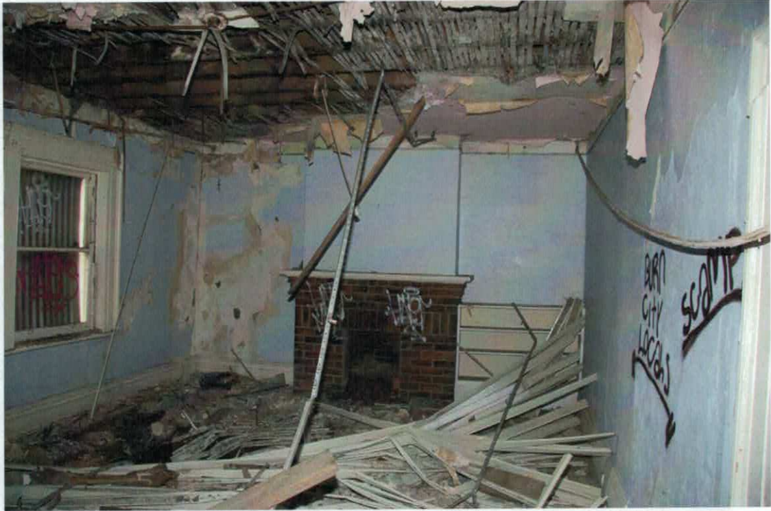
Figure 13 The main 'sitting room' on the first floor. Both the ceiling and floor are in a state of collapse.
