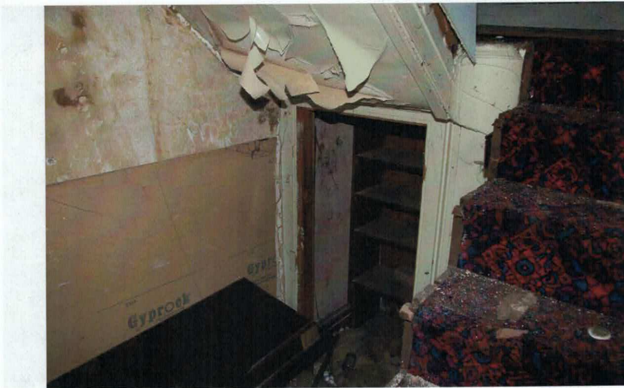
Figure 11 The central stair at ground level with missing balustrade.
