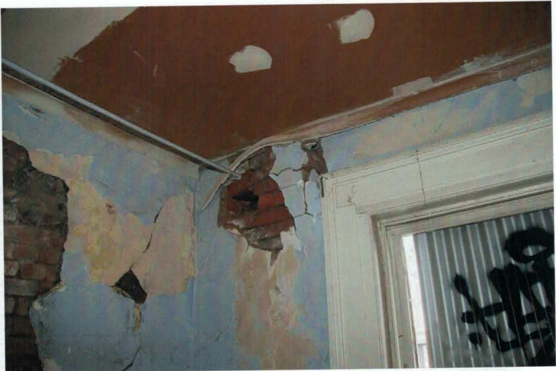
Figure 16 The typical architrave detail to doors and windows. Note the bulging bricks caused by wall movement.
