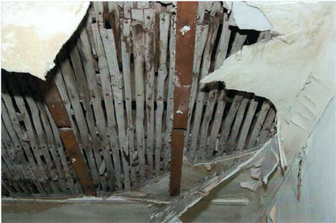
Figure 18 Split hardwood laths used in a ceiling. These are typical for the date of construction.
